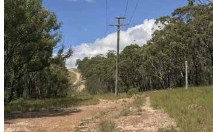
Existing overhead services
